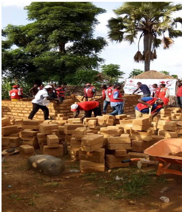
Nigeria Red Cross Society's community volunteers building a model house with bricks and materials provided by the Operation in Gombi, Adamawa State. Fifteen communities will receive two model houses each with technical skills developed to construct such houses. Many more houses will be built in the next phase of the Operation in 2018. Source: IFRC
