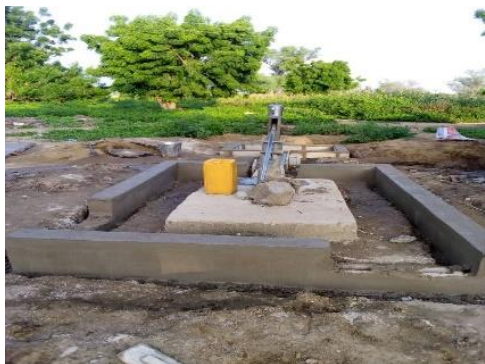
14 water points have been rehabilitated in five communities. Here in Song. Source: NRCS
